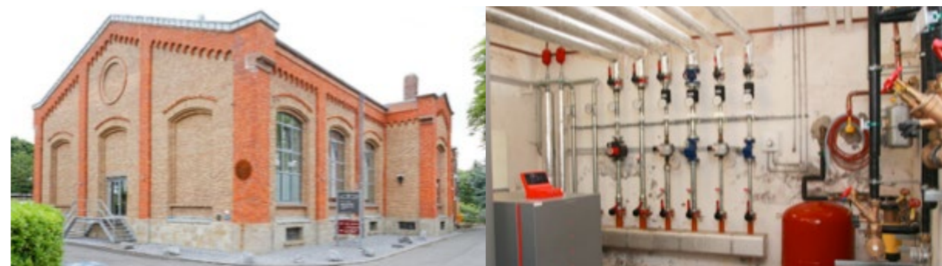
Figure 18: Old pumping station Haan – heat pump with ice storage in a reutilised non-residential building
