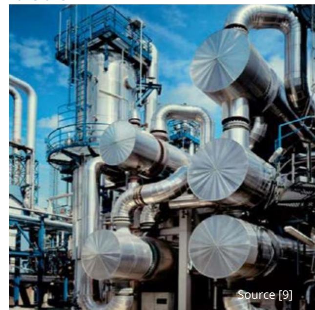
Figure 52: Heat exchangers at an industrial facility in Karlsruhe
