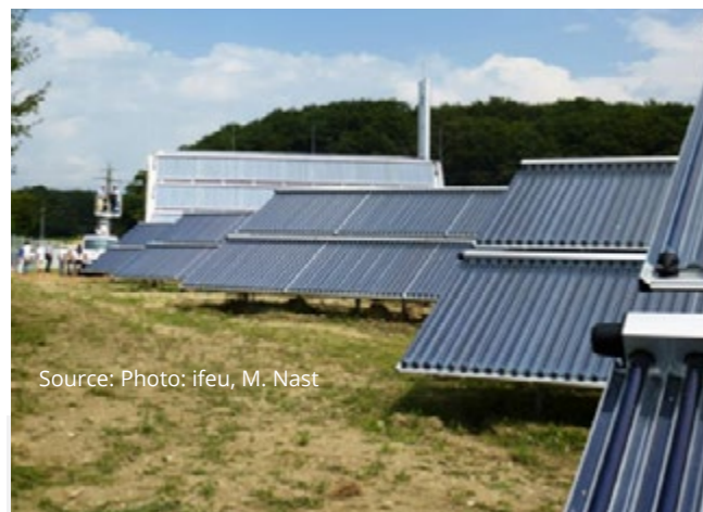
Figure 38: ETC collectors in the field in Büsingen
