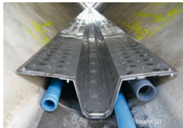
Figure 27: Sewage canal heat exchanger in Bretten
