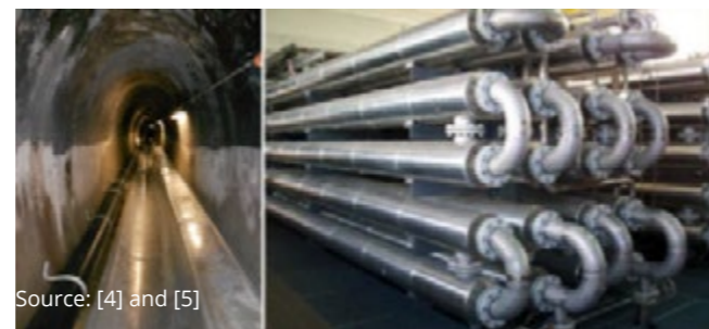
Figure 24: Sewage canal heat exchanger (left) and bypass heat exchanger (right)
