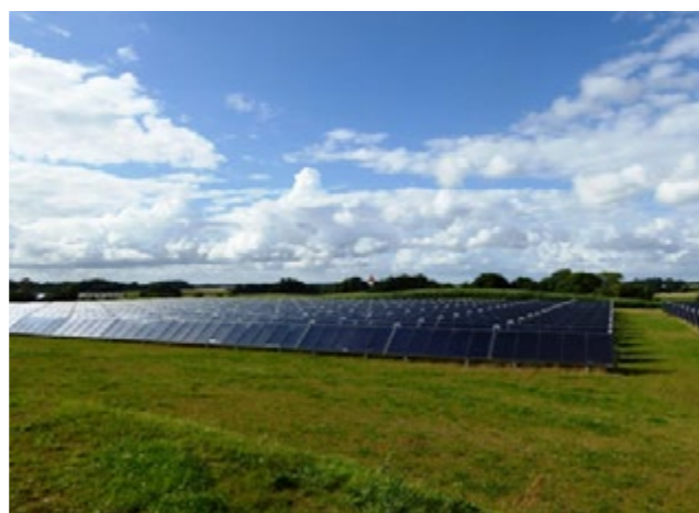
Figure 40: FPC collectors in the field near Dronninglund
