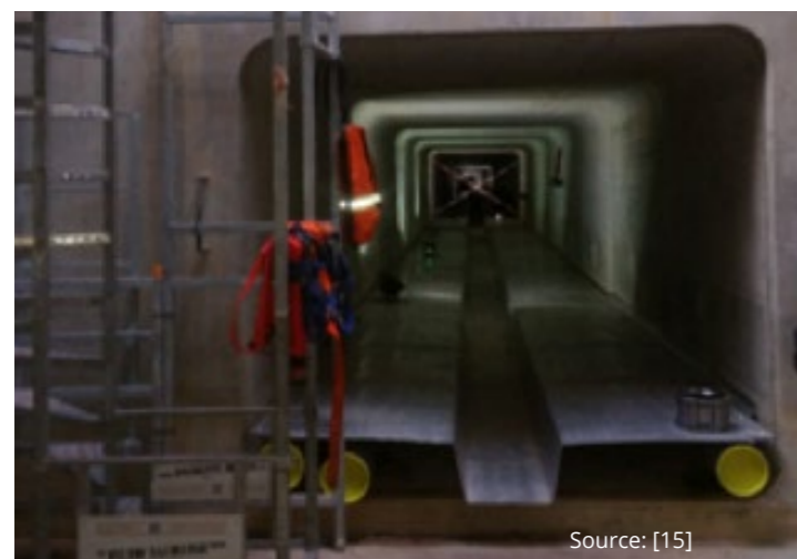
Figure 28: Sewage canal heat exchanger in NeckarPark
